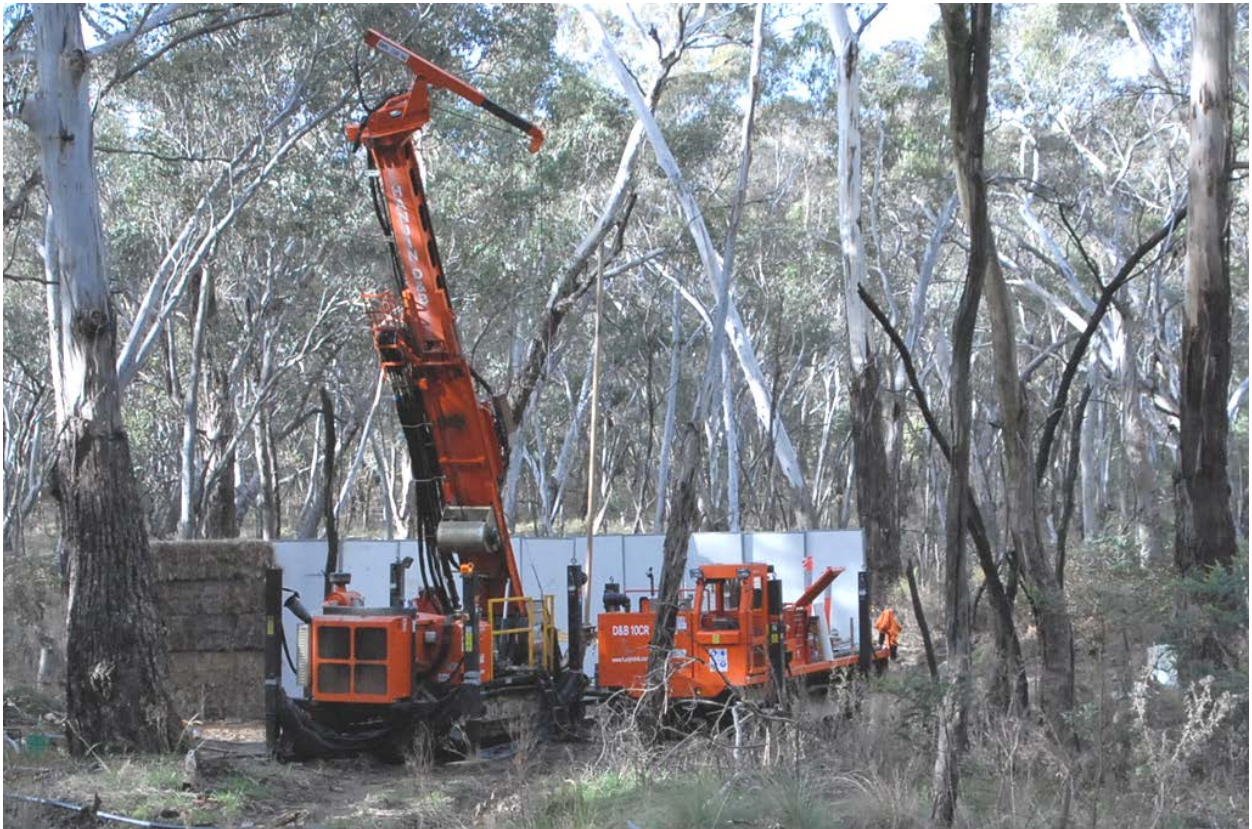
Track-mounted Hanjin 7000SD drill machine at North Big Nugget Hill. Hay bale and reflective sound screens behind the drill pad are used to reduce the sound impact of drilling for the residents of Hargraves Township.
