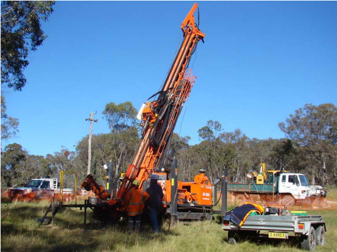
Track-mounted Hanjin 7000SD drill machine on site at Hargraves North Big Nugget Hill.
